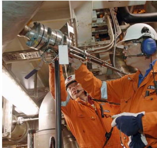
Figure 3: Inspection of inline sensor probe (Photo: StatoilHydro).
